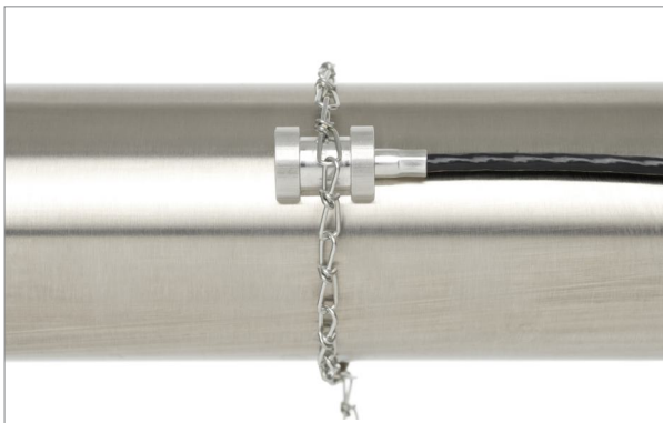
Pt 100 transducer fixed to pipe
